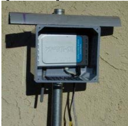
Figure 2-7: Enclosing an AP within a NEMA Box
