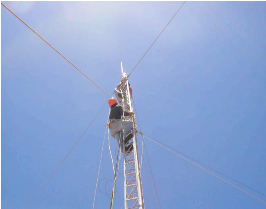
Figure 7.2: A climbable guyed tower.
